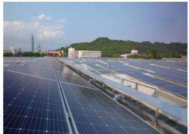
▶ Solar photovoltaic system installed in water.
