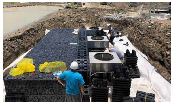
► Rainwater tank at Hsinhsin Park.
