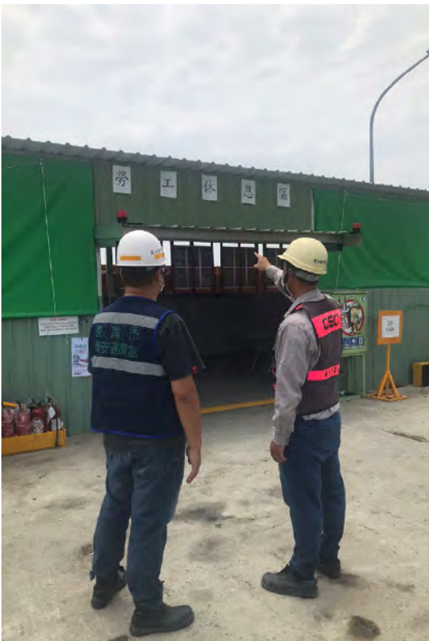
△ Heat Hazard Site Inspection
