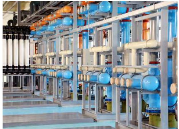
△ RO Reverse Osmosis Equipment in Anping Water Reclamation Plant
