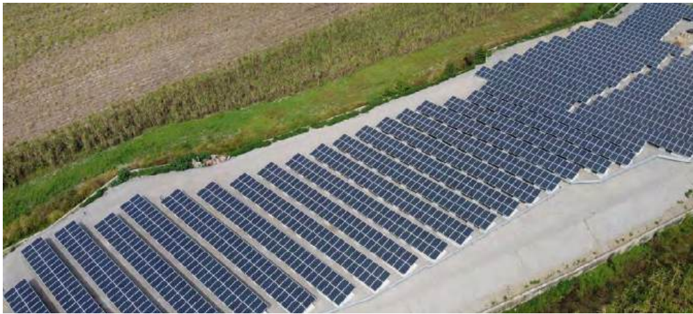
△Houbi District Jingliao Landfill Power Plant
