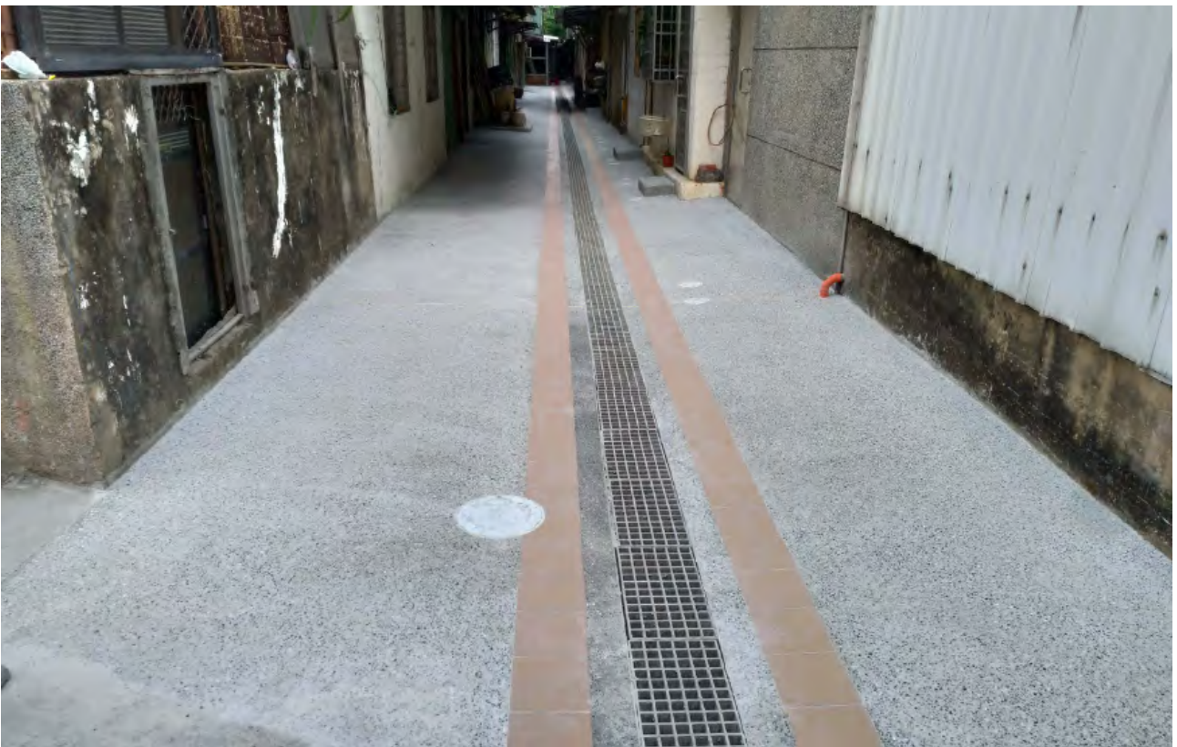
△ Waste Water Sewer
