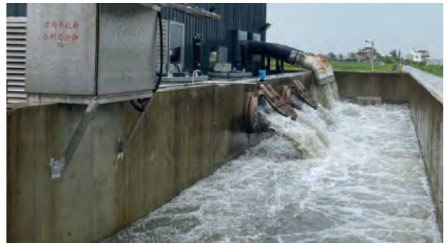
△ View of the Pumping System of the flood storage pond in operation
