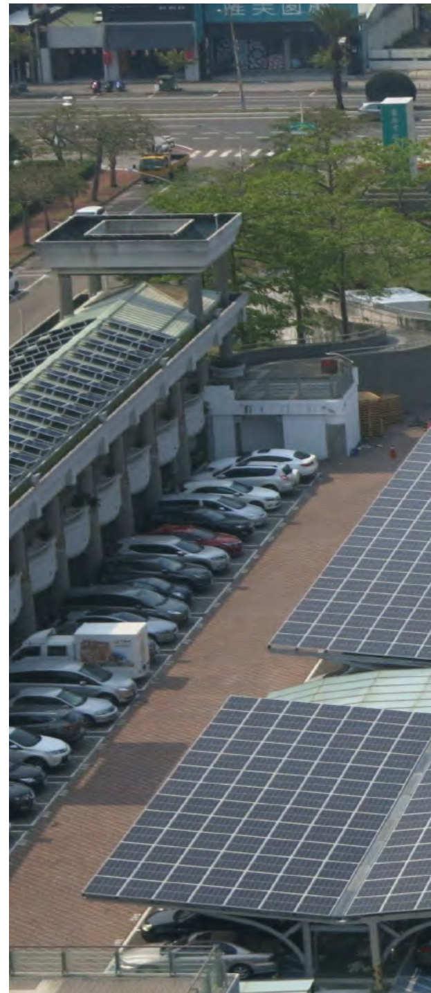
Solar Panel Roof in the Parking Lot of Yonghua Civic Center
