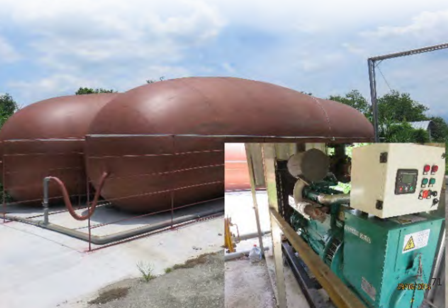
▼ Equipment for biogas power generation
