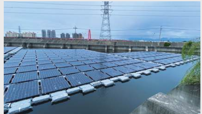
▲ Detention pond floating solar photovoltaic in Wuri HSR
