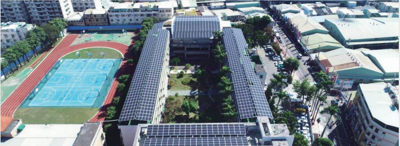
▲ Photoelectric installation on the roof of Taichung City Zhongping Junior High School
