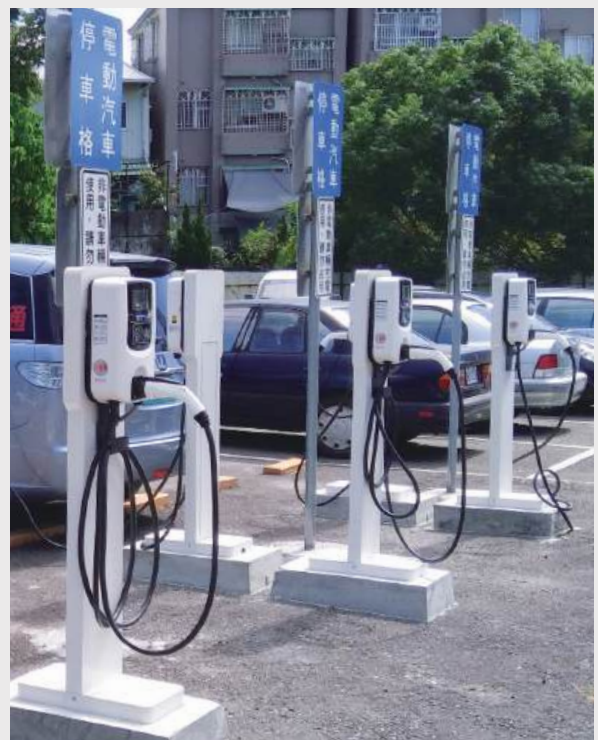
▲ Electric vehicle charging equipment in the second parking lot of Yangming building
