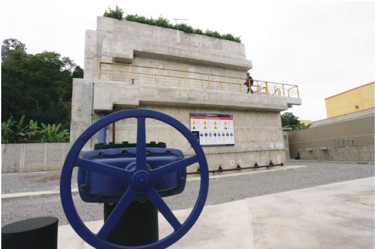
Sewage Treatment Plant (ETE) Maria Paula.
