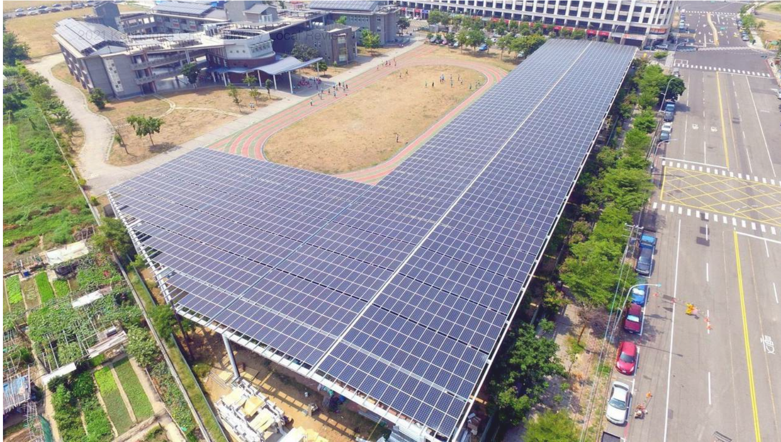
▲ Photovoltaic projects on campuses
