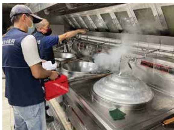
Technical instrumentation to confirm front-end hood performance
