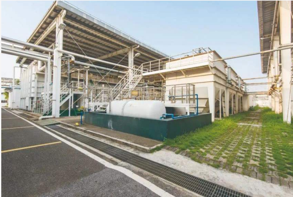
The GAC Honda wastewater treatment plant
