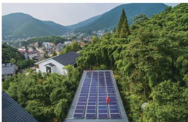
Fig. 2-14 Deqing Rural Rooftop Photovoltaic Installation
