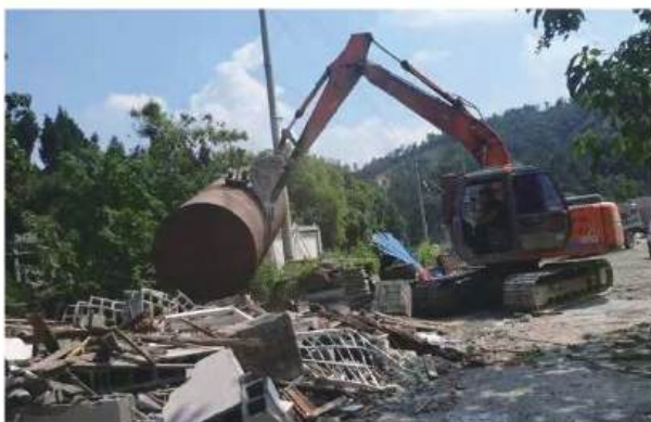
Fig. 2-16 Elimination of Outdated Production Factory
