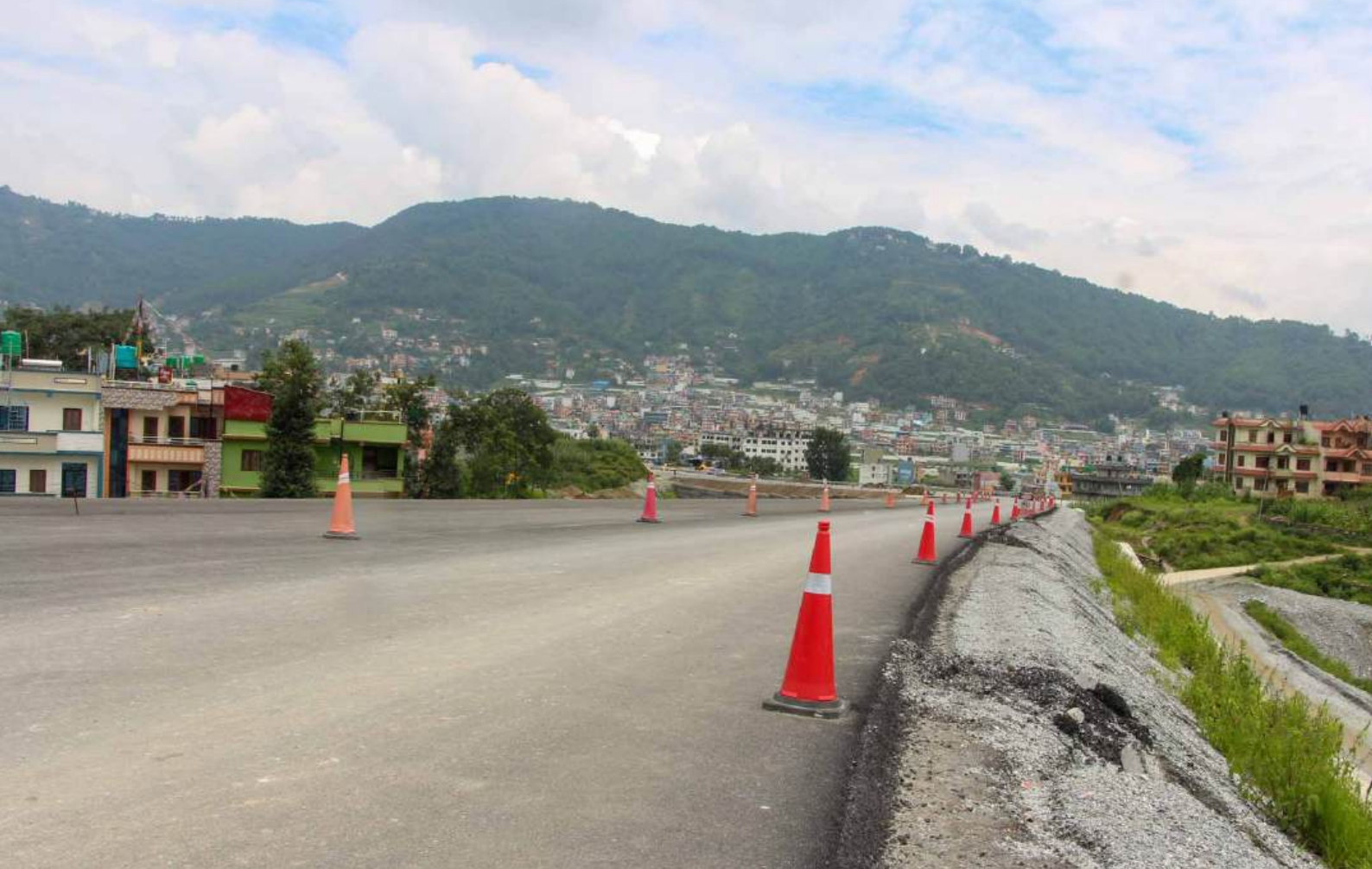
Connectivity and safer mobility are a key concern of Chandragiri Municipality © UN-Habitat, 2024
