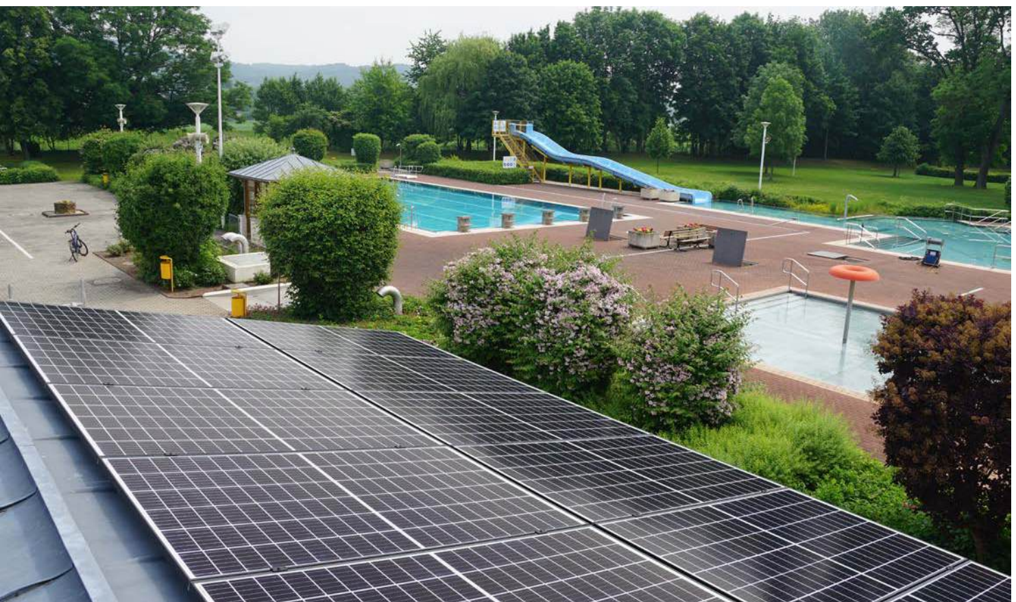
Photo 15: Photovoltaic system on the roofs of the buildings of the leisure and recreation baths © Stadt Bad Köstritz
