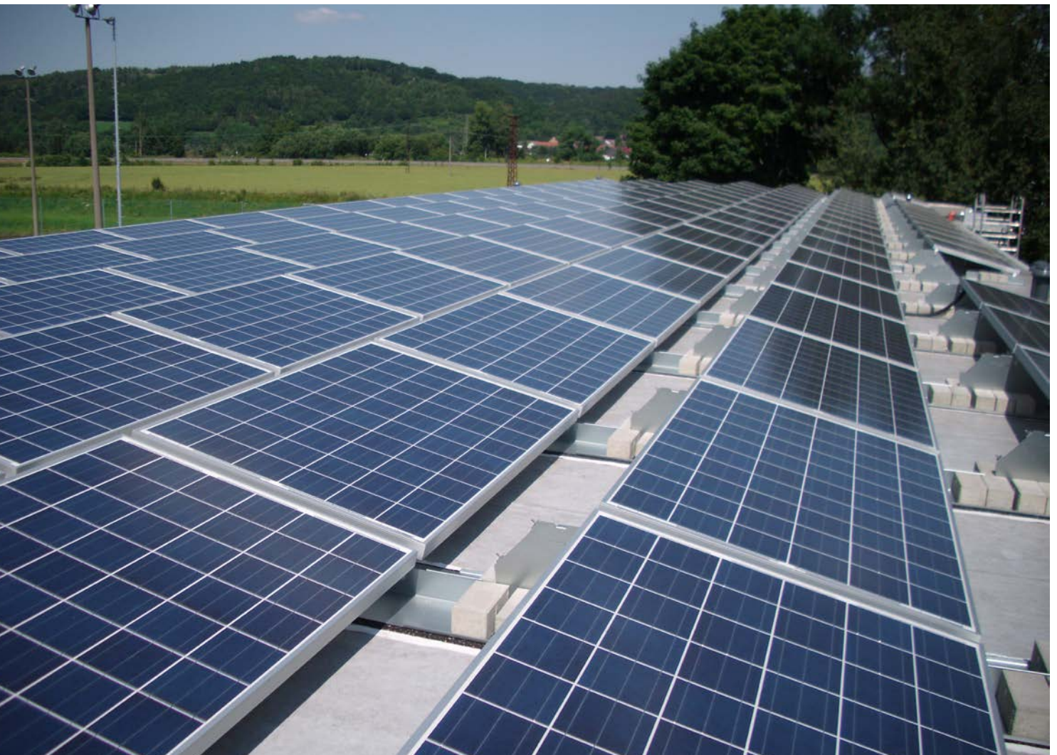
Photo 16: Photovoltaic system at the sports field "Am Drehling" © Stadt Bad Köstritz
