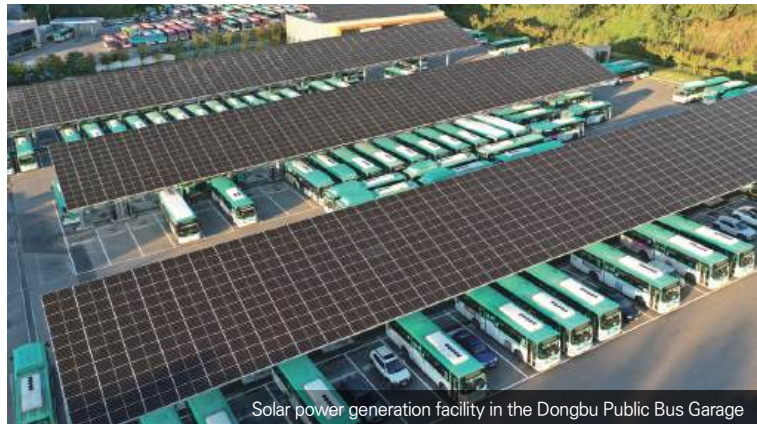
Solar power generation facility in the Dongbu Public Bus Garage
