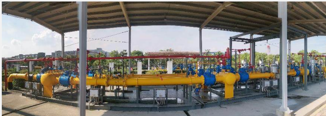
Figure 8 Natural Gas Station of Pu'nan Area in Songjiang
