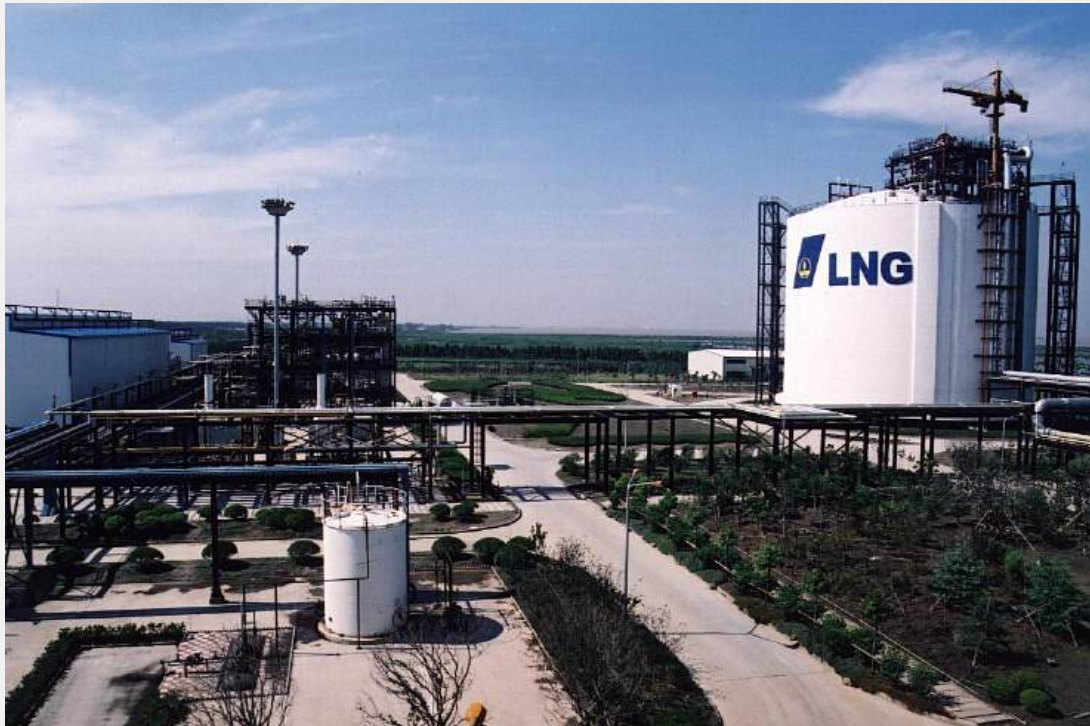
Figure 11 LNG Terminal in Wuhaogou, Pudong New Area
