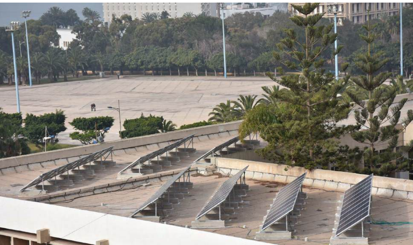
Figure 19. PV Hotel de ville. Source: Municipality of Agadir (2023)
